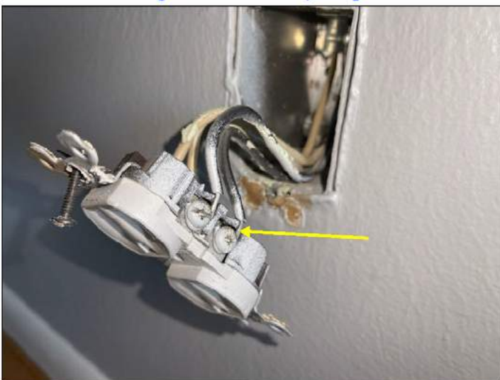
Aluminum wiring Outlet on the west wall of the front room
