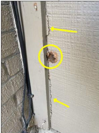
Minor damage to the siding east side of the home by the back garage door
