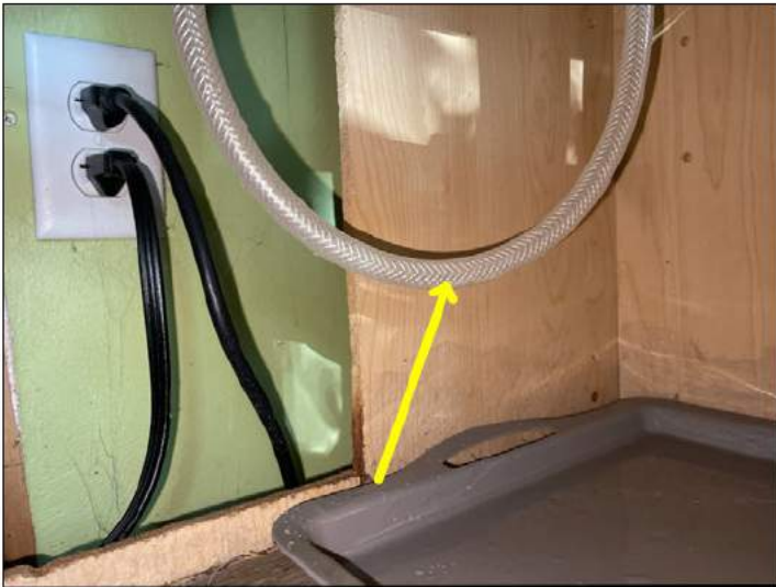
Connection to the sprayer is leaking
