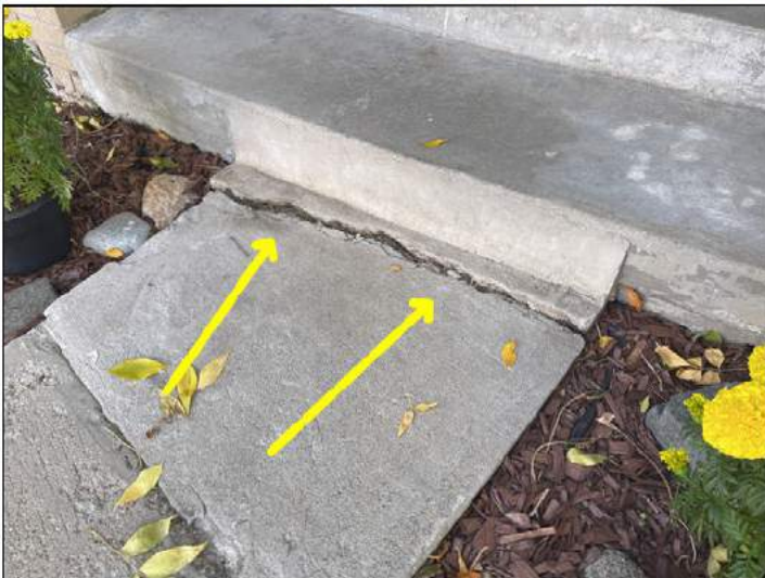
Cracking and settling in the front
