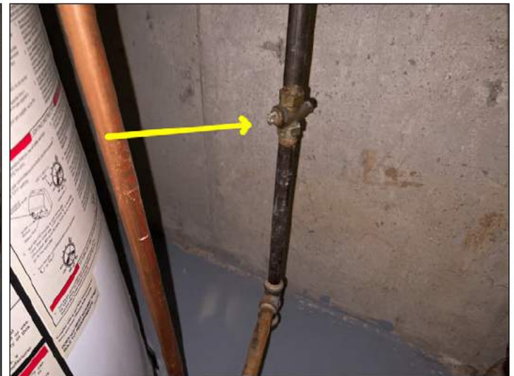
Gas shut off to the water heater
