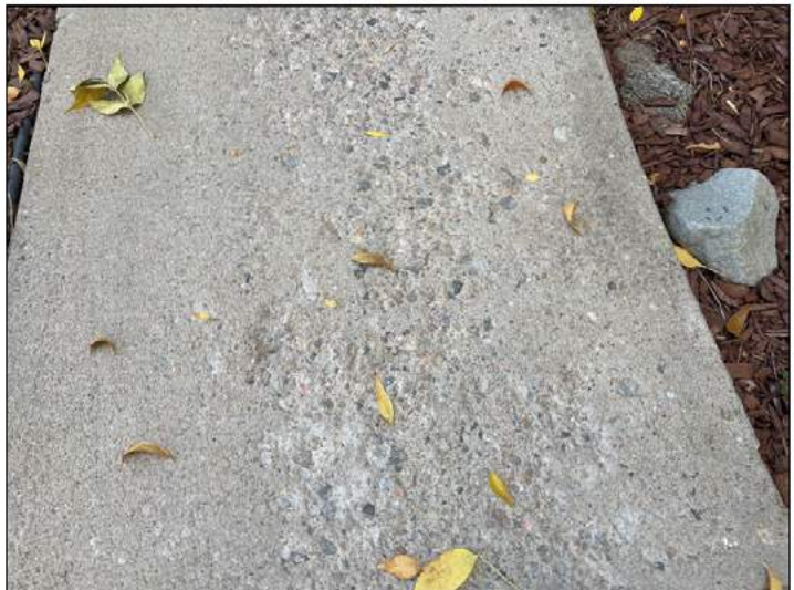
Spauling at the front walkway
