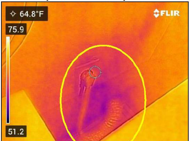
Dark blue is moisture in the drywall
