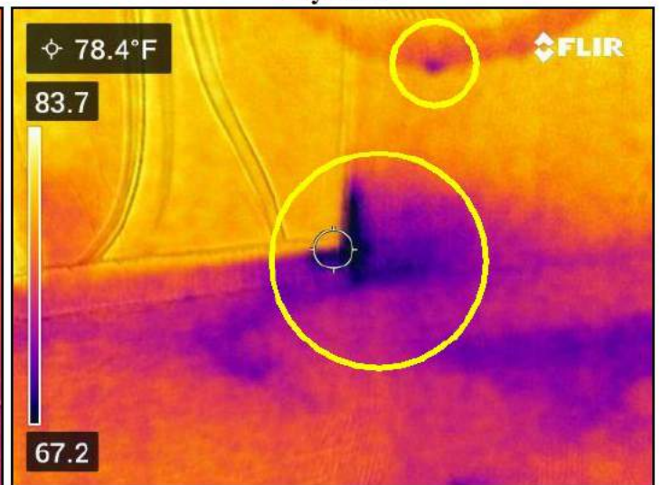
Moisture from the leak at the sprayer
