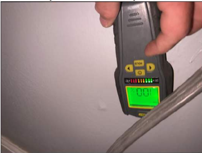
Moisture meter showing moisture in the drywall of the laundry room
