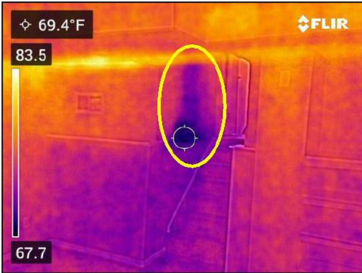
Moisture in the basement wall at the stairs
