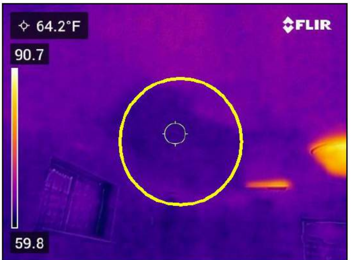
Moisture in the basement ceiling
