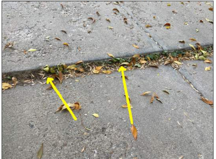
Settling on the driveway
