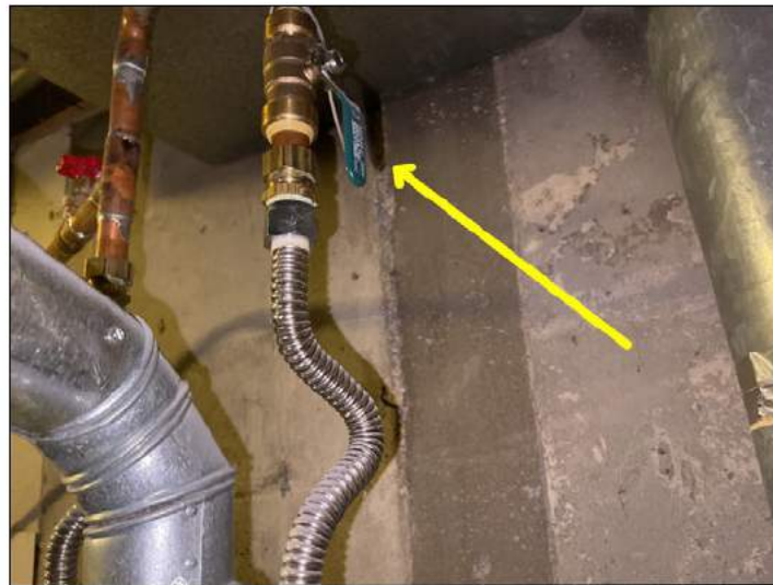
Water shut off to the water heater
