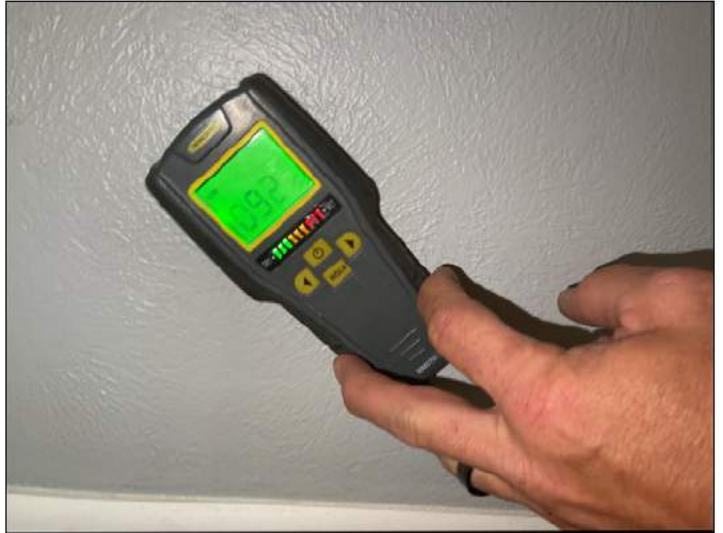
Moisture meter showing moisture in the drywall
