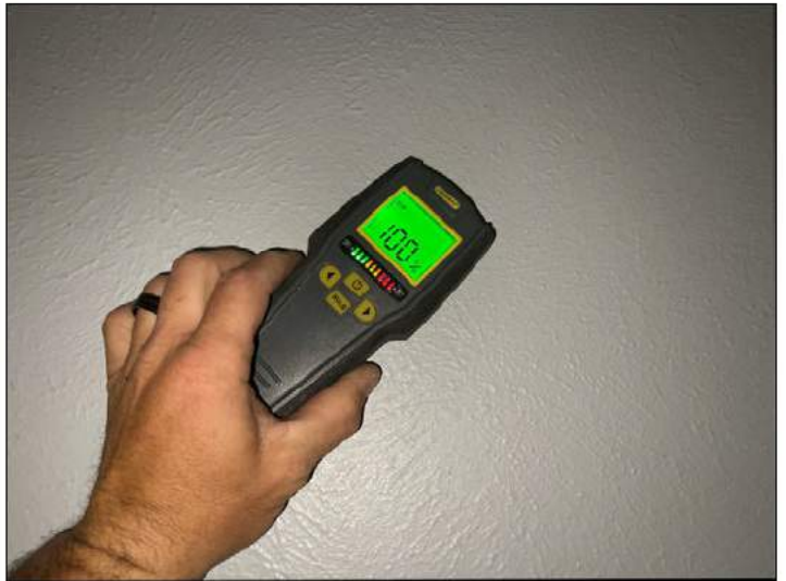
Moisture meter confirming moisture meter in the wall
