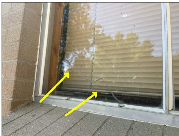
Cracked window pane east side of the home
