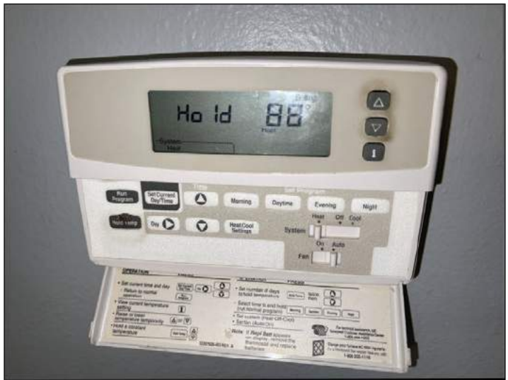
Thermostat setting to test heat
