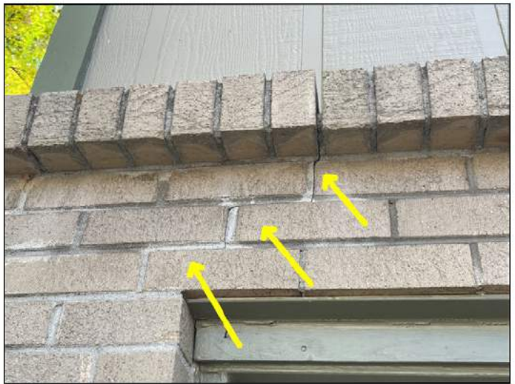
Monitor minor settling crack front east side of the home above the east garage door
