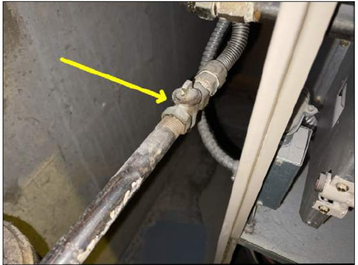
Gas main shut off
