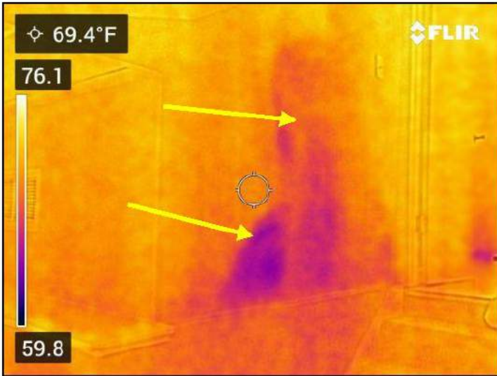
Basement wall showing moisture in the drywall
