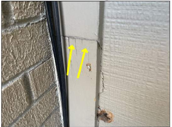
Seal gaps at the trim east side of the home
