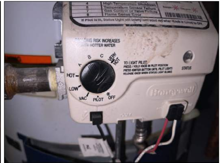
Water heater test setting
