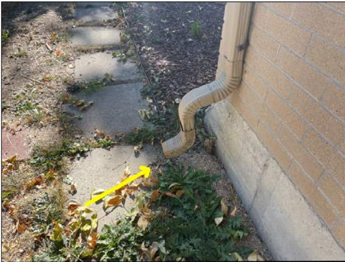
Missing extension on the east side of the home
