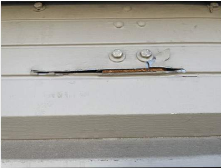
Minor damage to the top of the west garage door
