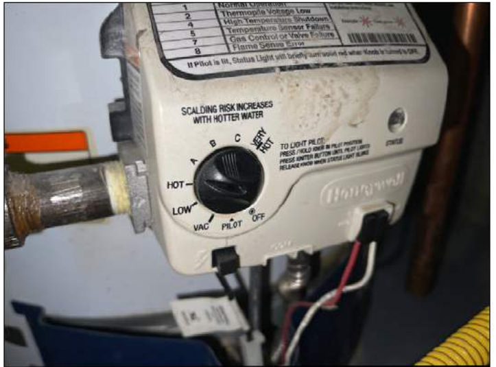
Water heater return to initial setting
