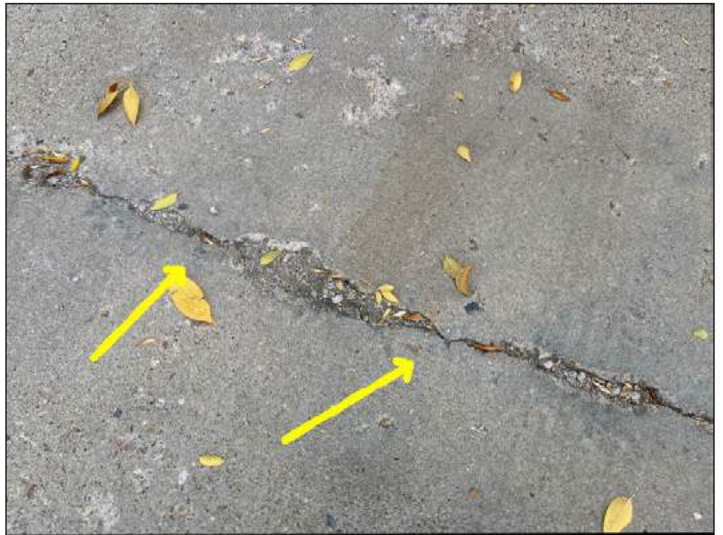
Cracking in the driveway
