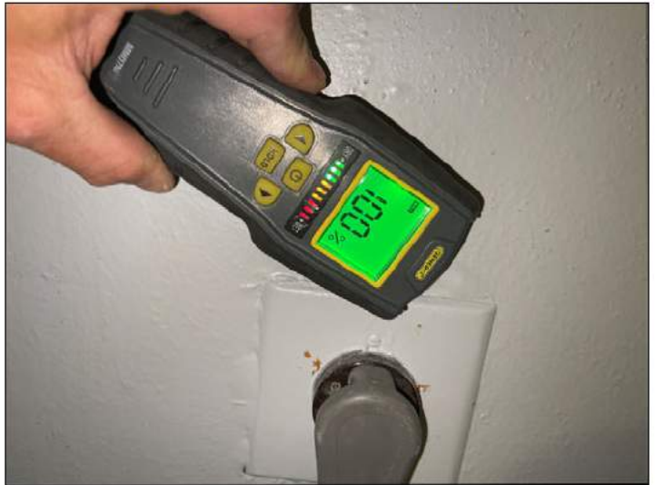
Moisture meter showing moisture in the drywall of the laundry room
