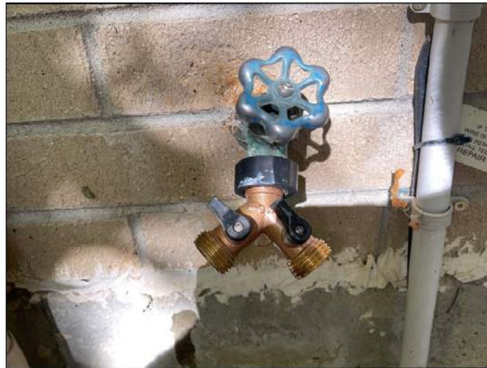
Faucet at the back is not on
