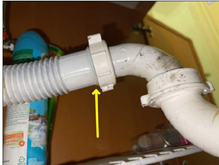
Leak at the connection
